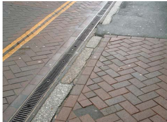
Poor quality existing floorspace
