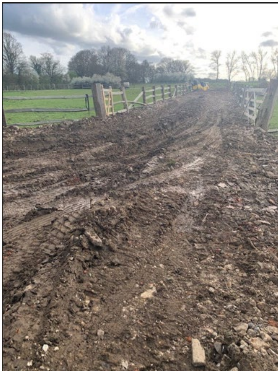
At the entrance to the Land from Rosemary Lane looking south into the Land with where the access has been widened and a hardsurfaced trackway leading into the Land beyond the gates
