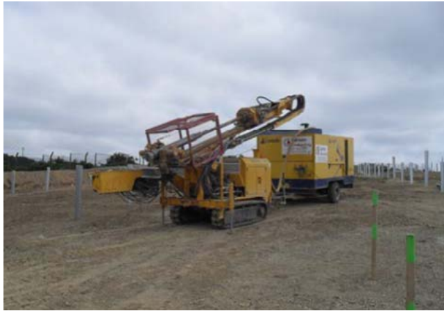
Where pile driven foundations are proposed consideration should be given to the noise impact at nearby sensitive receptors. Difficult ground conditions, such as those encountered at the 1.4MW Wheal Jane solar farm shown here, may also require drilling.
