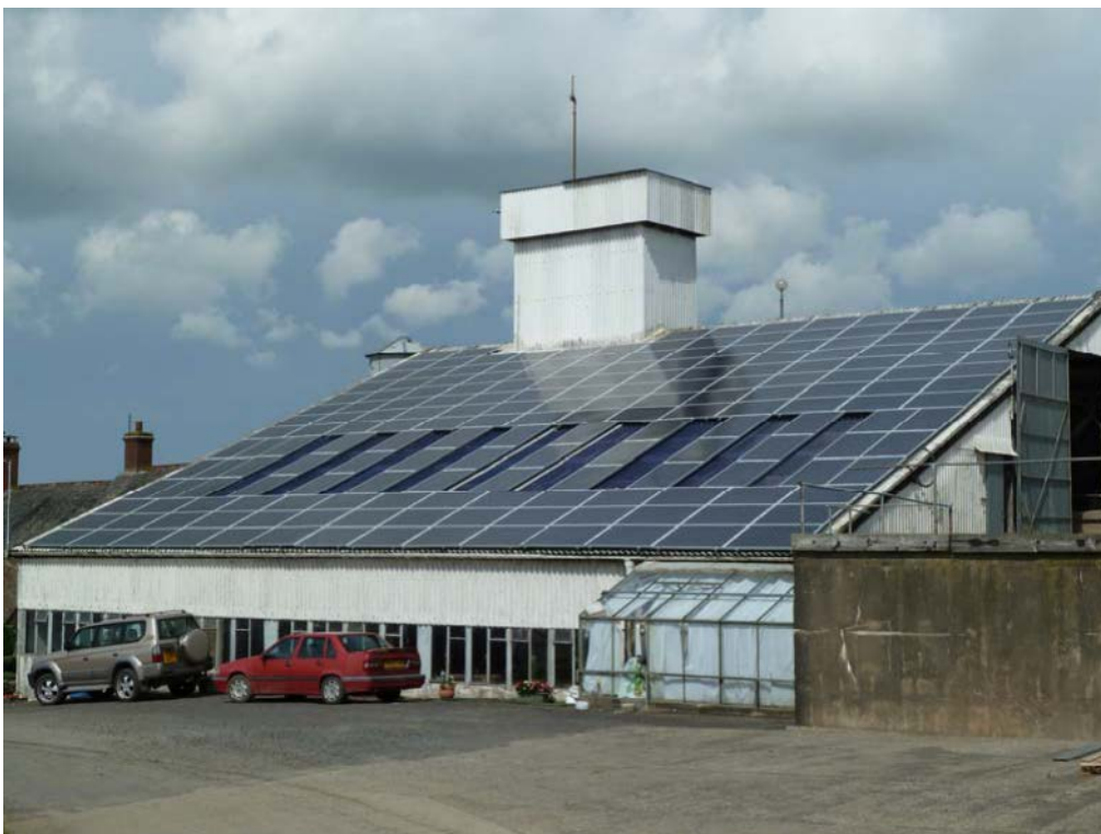
The roof of this agricultural grain drying unit has been clad with solar PV panels which generate a high proportion of the electricity required by the facility. Image courtesy of Clean Earth Energy
