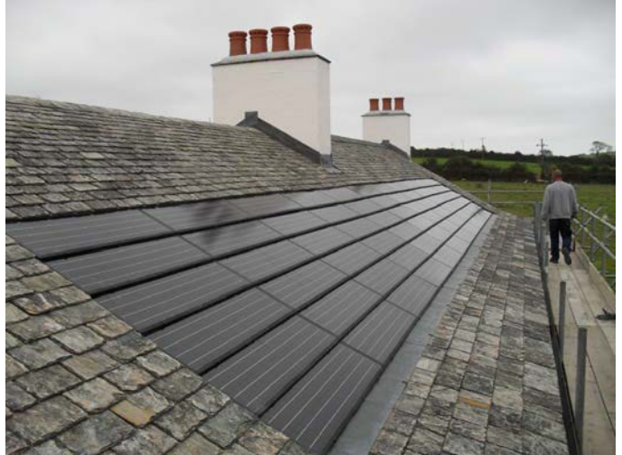
A roof mounted 4kW solar PV installation being installed while the roof is being re-slatted
