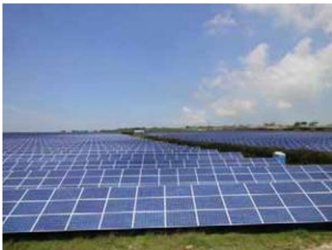
The 5MW Trefullock solar PV farm, Cornwall
