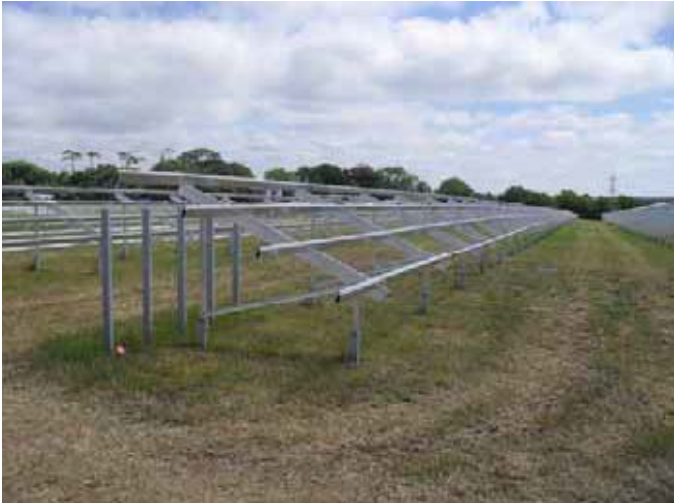
The ground anchors and framework associated with the development of the 1.4MW Benbole solar PV farm in Cornwall
