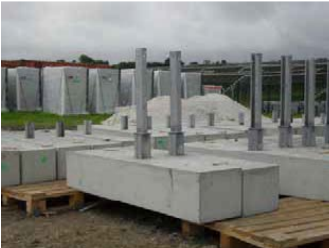
Where there are areas of archaeological interest, and therefore a need to avoid ground disturbance, the use of pre-cast concrete anchors should be considered, as shown here at the 5MW Trefullock solar PV farm in Cornwall
