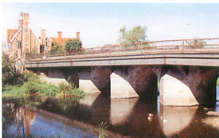
Above: The sturdy 17th century bridge, albeit with a 20th century decking, continues to carry traffic over the river.
